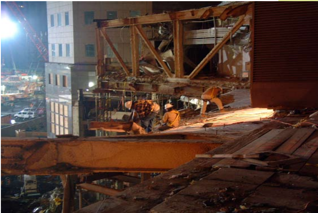
Workers Clearing Debris at Heights >30 Feet
